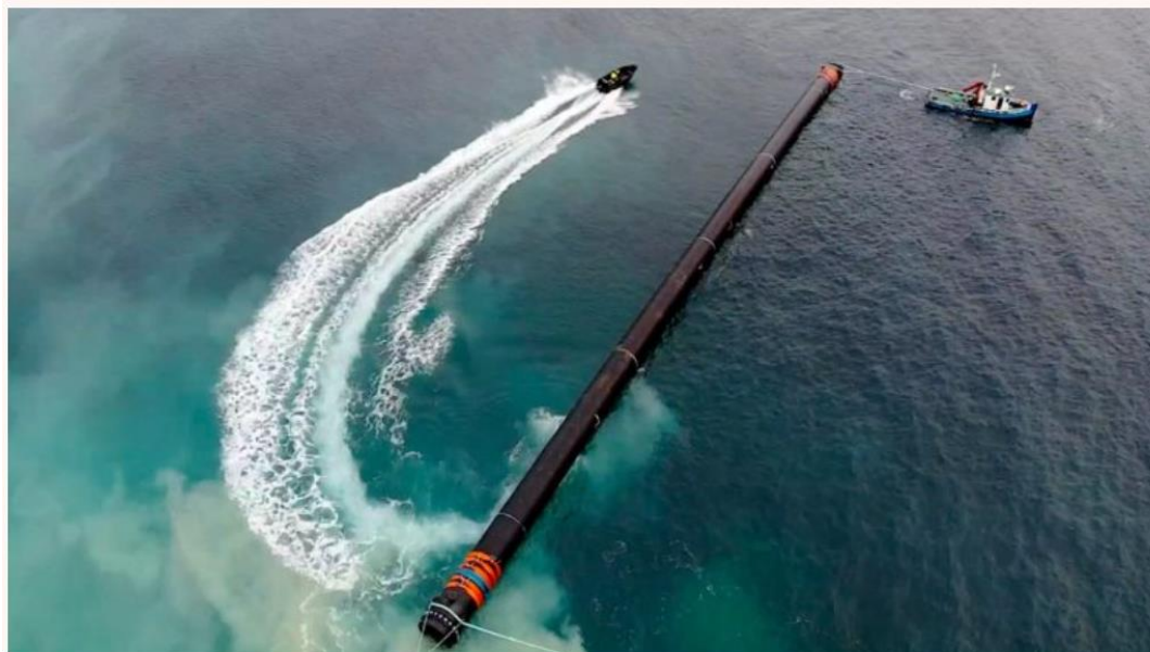
One of the inlet pipe from Andfjord Salmon's large land-based fish farm on Andøya, Northern Norway, PHOTO: Andfjord Salmon
